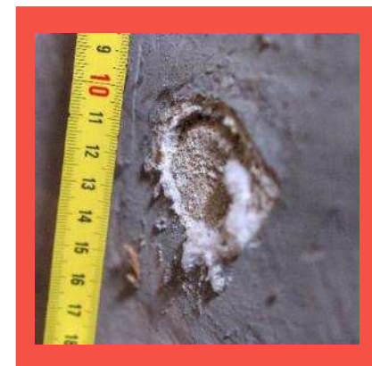
salt efflorescence nitrates and sulphates
